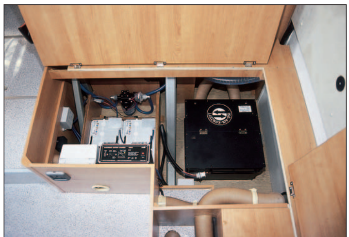
The space under the lounge seats is given over to the twin batteries, RCD, pump and ISO cooling unit, amongst other things. Everything is easily available for servicing and although there is little storage space this is of little consequence given what is available elsewhere.
